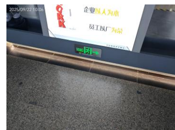
Evacuation direction sign.jpg
