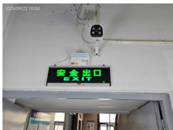
Emergency light and exit sign.jpg
